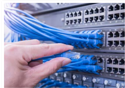
Plug & Play Unmanaged Switches
