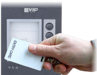
Gate Control via Card
