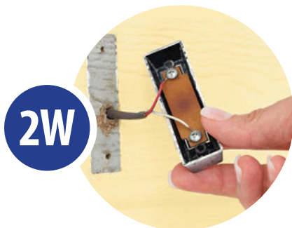
Upgrade Existing 2-Wire Systems
