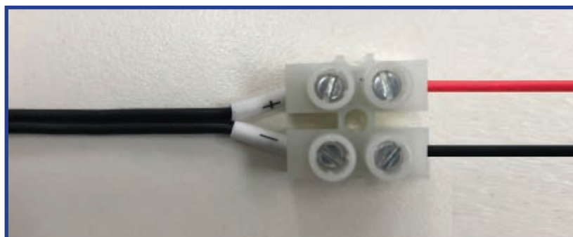
Fig. 2.3f Solar battery cables connected to terminal block
