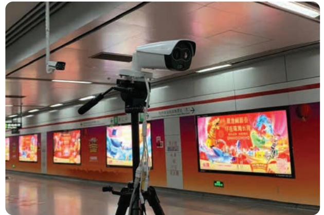
Example installation inside a train station
